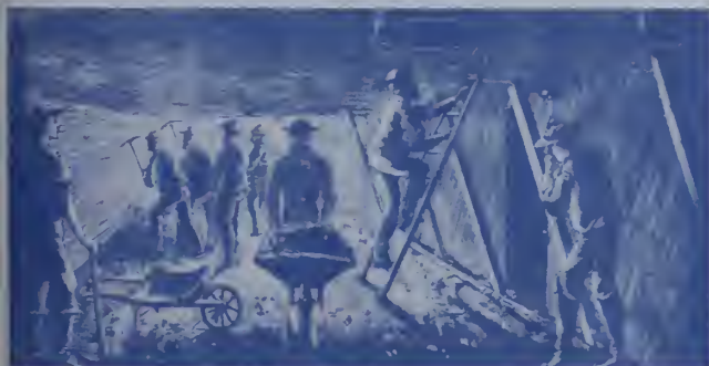
The men working under compressed air entered and left through air locks. Many were victims of "caisson disease." All together, the bridge claimed 20 lives.
